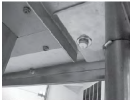
Figure 2-6 HHS Bolts Secured
