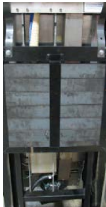
View of the counter-weights with cover removed
